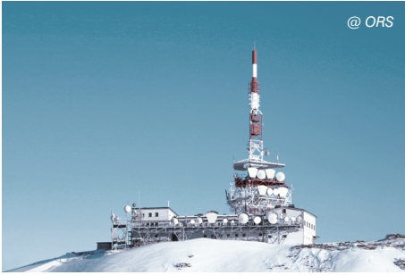
ORS operates nine modern large broadcasting Centres throughout Austria. The picture shows the Patscherkofel/Innsbruck transmitter.
